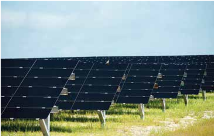
City of Tallahassee Solar Farm
