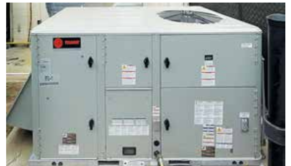
HVAC system upgraded at Lawrence Gregory Community Center
